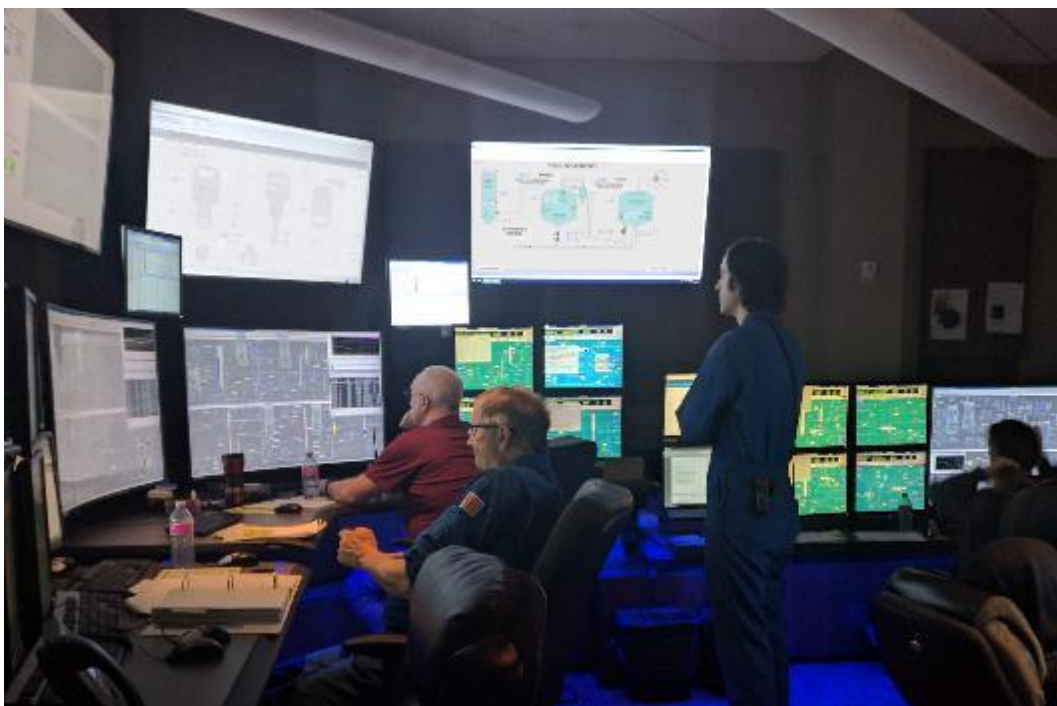
Figure 2. Another Simplified DCS screen for FCC standby operation at console
