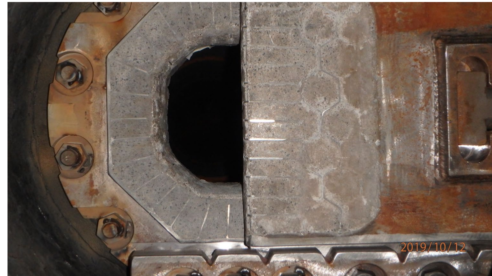
Slide Valve in Good Condition after Turnaround
