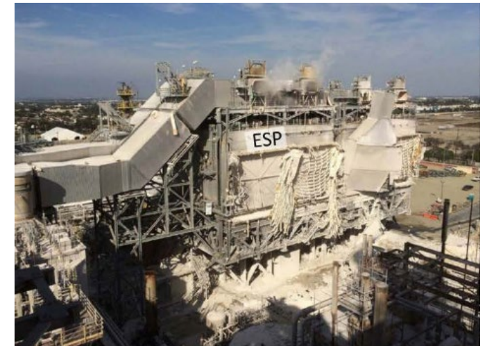
Torrance 2015 Incident: ESP Damage CSB Investigation Report, Figure 18
