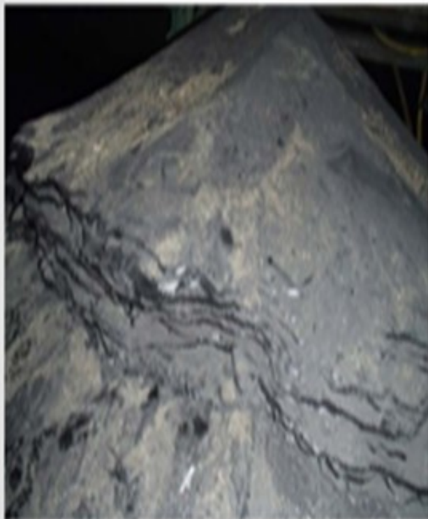
Deposits on Riser Termination Device
