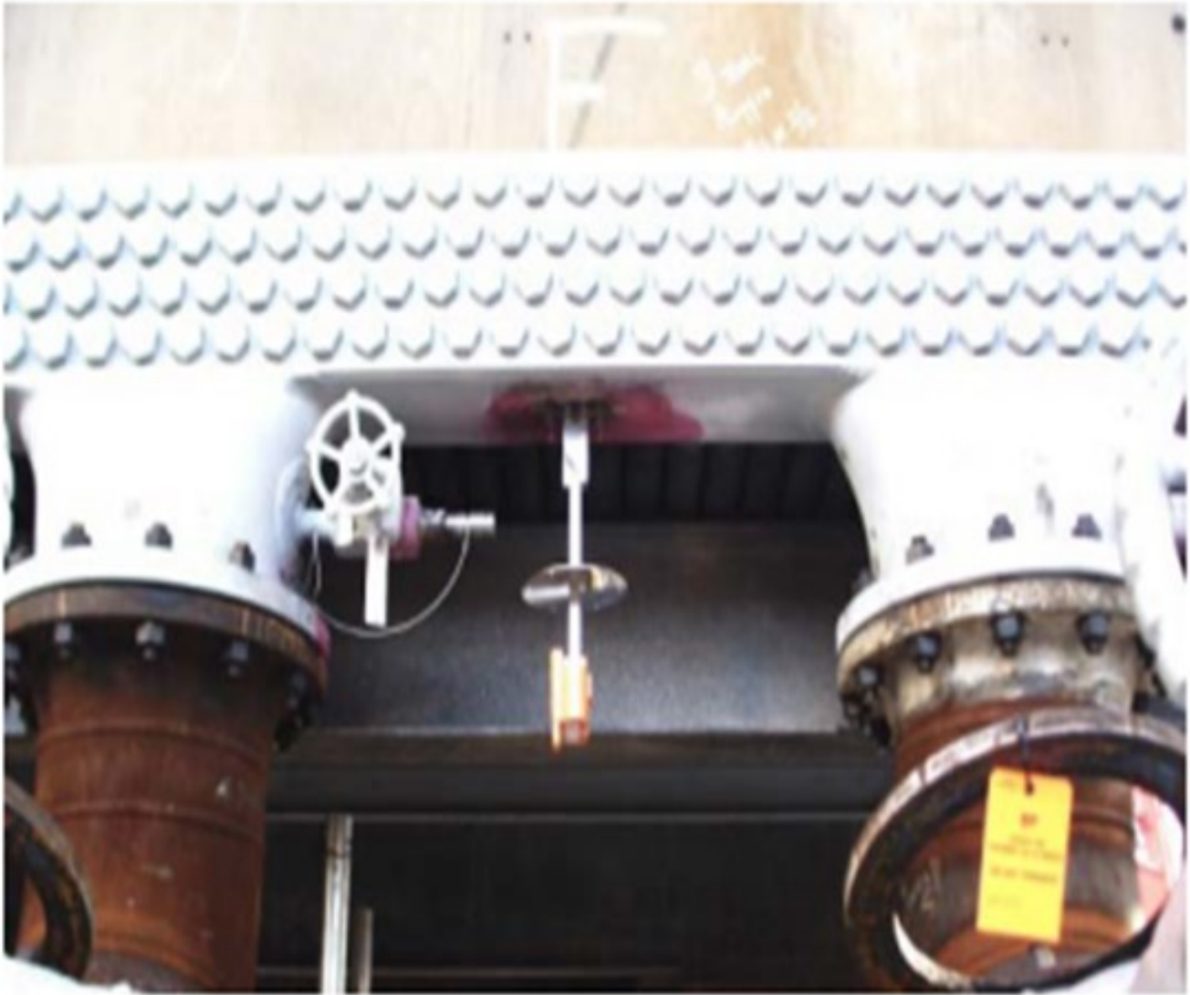
Permasense® UT probe on air cooler header box
