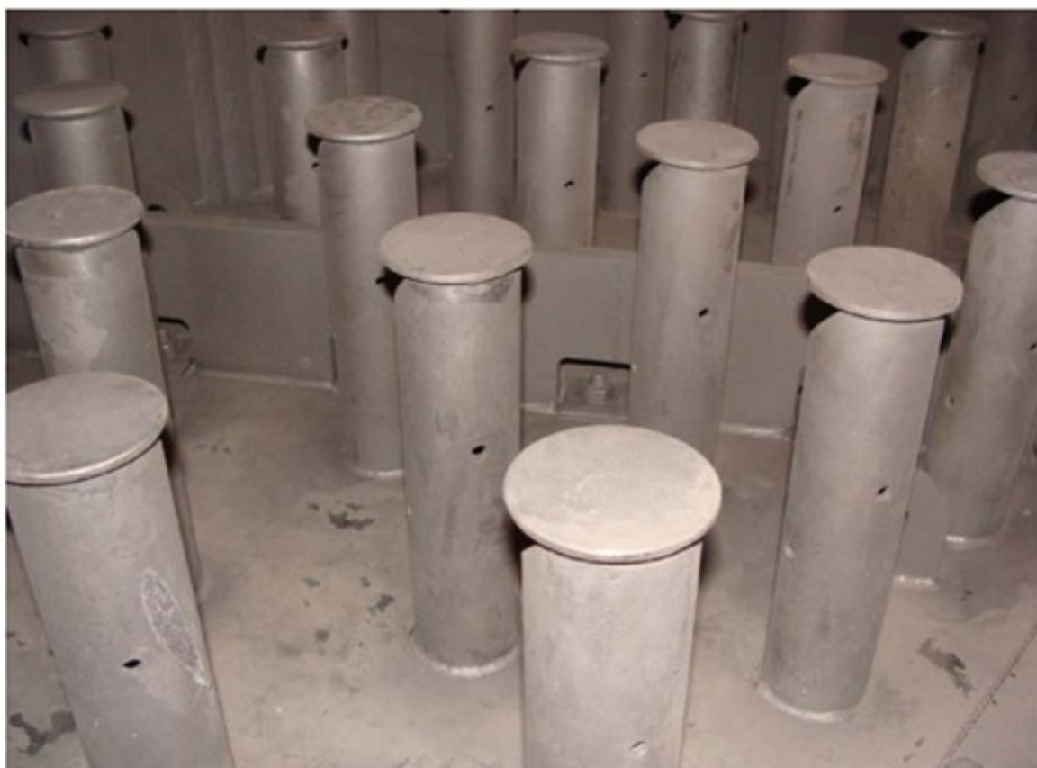
Top Tray Liquid Distributor – Overview after CO 2 Blasting
