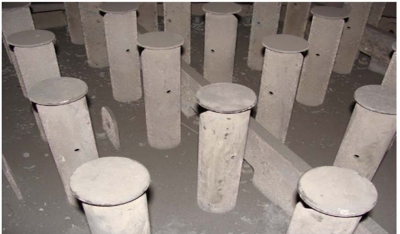
Top Tray Liquid Distributor – Overview prior to cleaning
