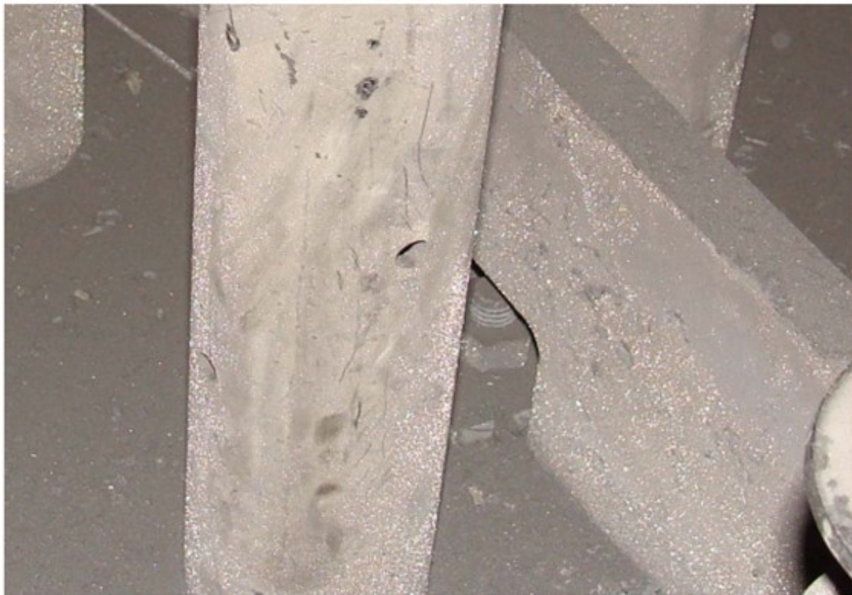
Top Tray Liquid Distributor – Close up of scale prior to cleaning
