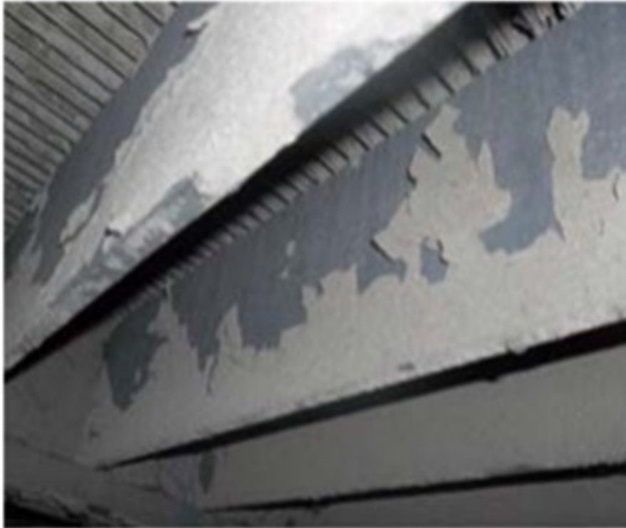
Reactor Catalyst Support Deck – Underside Scale
