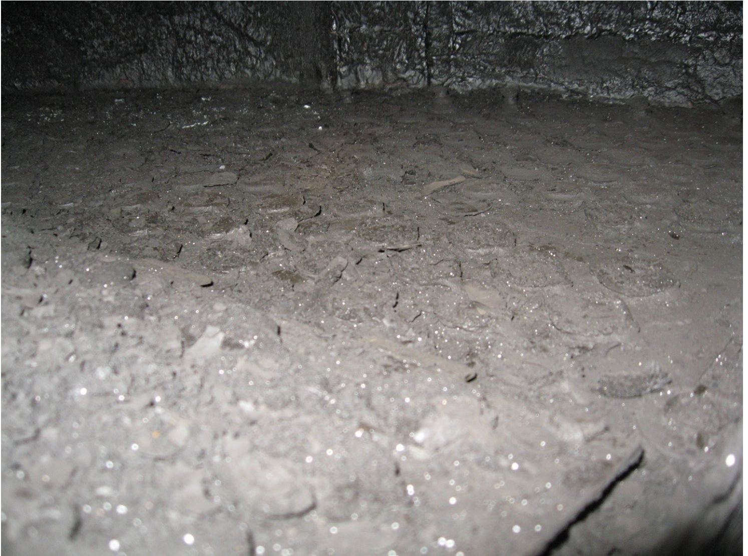
Figure 2. Barium fouling in wash section of atmospheric crude tower
