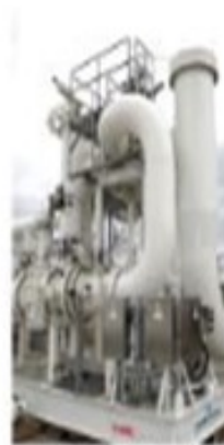
Crude Custody Transfer Skid
