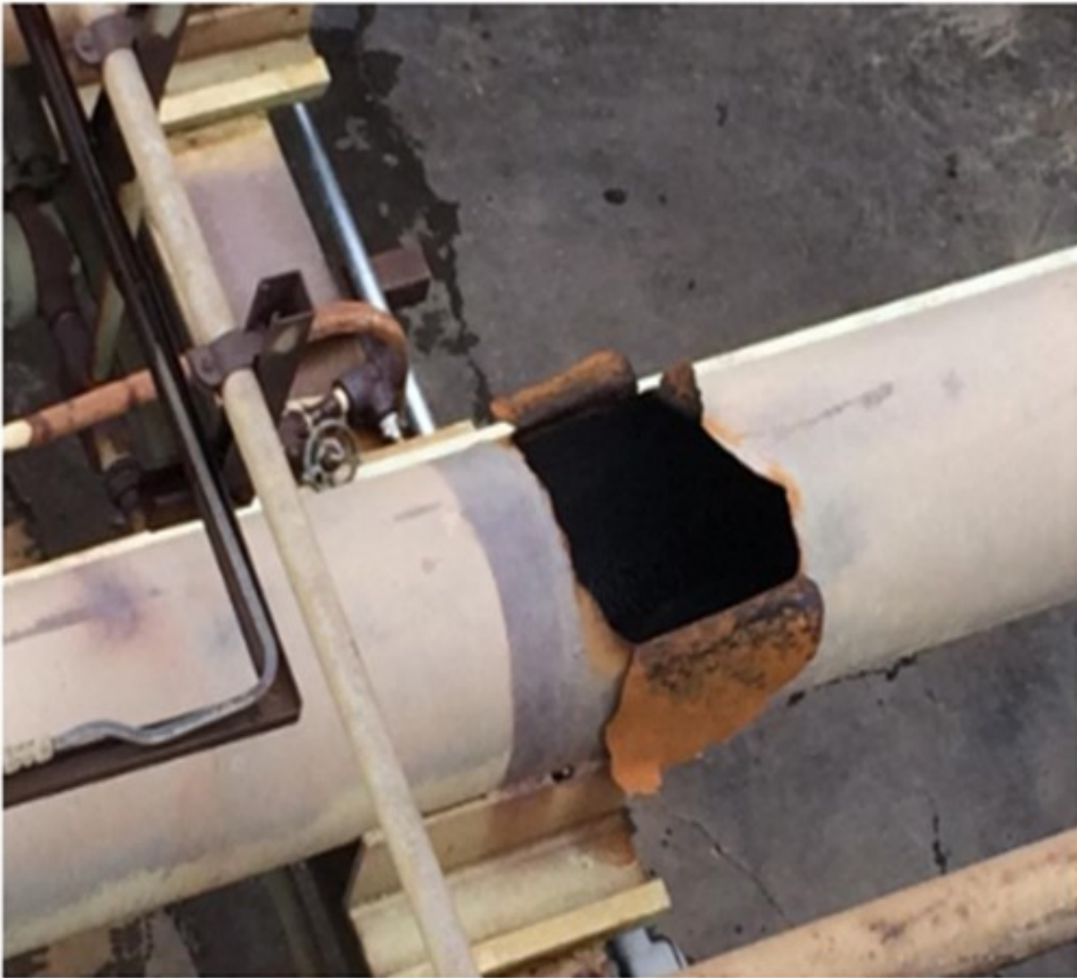
Figure 1. Reactor Effluent Piping Failure at MPC NHT
