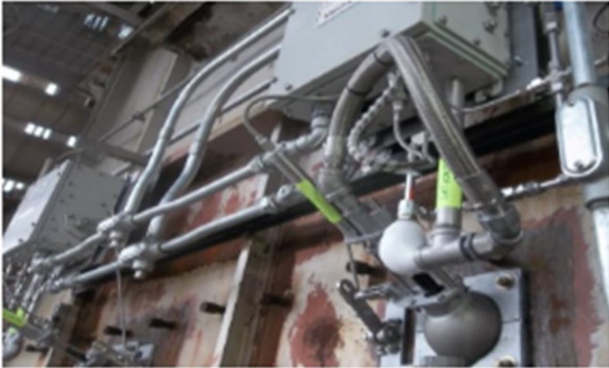
Figure 3: TFM installation on older SMR
