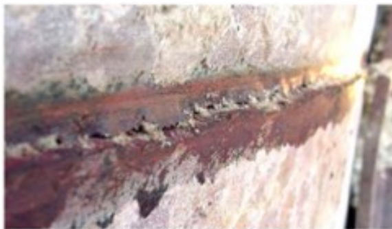
Circumferential weld seam cracking
