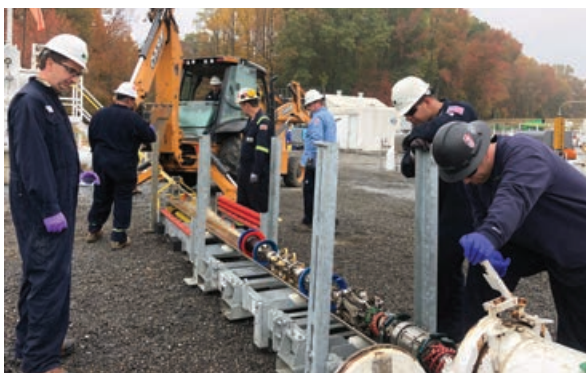
MIPC uses an In-line inspection tool (ILI) or also known as a smart pig. An example is a magnetic flux leakage (MFL). MFL pigs use strong magnets to detect disturbances in the magnetic field that are caused by defects. The relative size, shape, and location of the defects can then be determined and used for repair planning (Pre-COVID picture).
